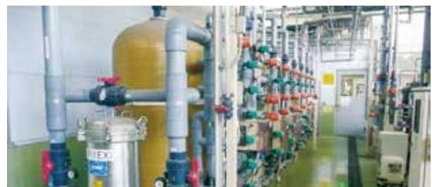
Ion exchange tower
