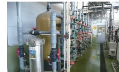
Ion exchange tower
