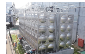
Batch type final effluent tank
