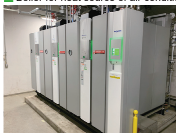
Boiler for heat source of air conditioning
