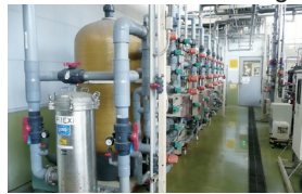
Ion exchange towers
