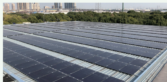
Mega solar panels which were introduced in TRCW (China) (Installed in FY 2017)
